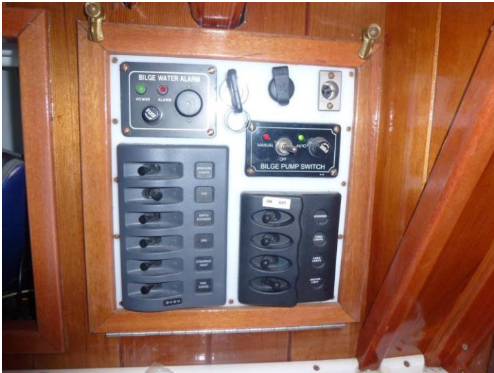
Switchboard, bilge and high water alarm.
